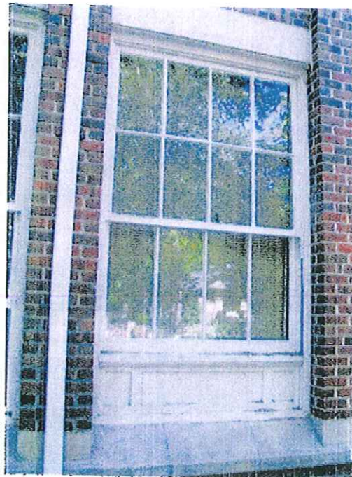
Figure 132: Exterior view of window type F. Note the wood paneled area in the lower portion of the lower sash.
