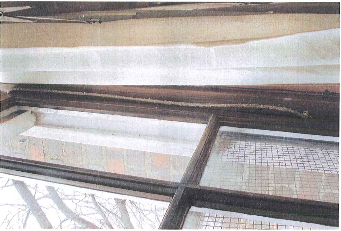
Broken sash cord, West Classroom, 2nd Grade
