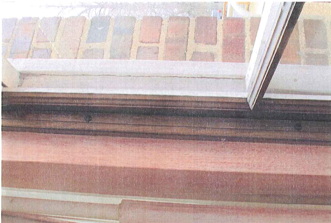
Paint cracking on exterior West Classroom
