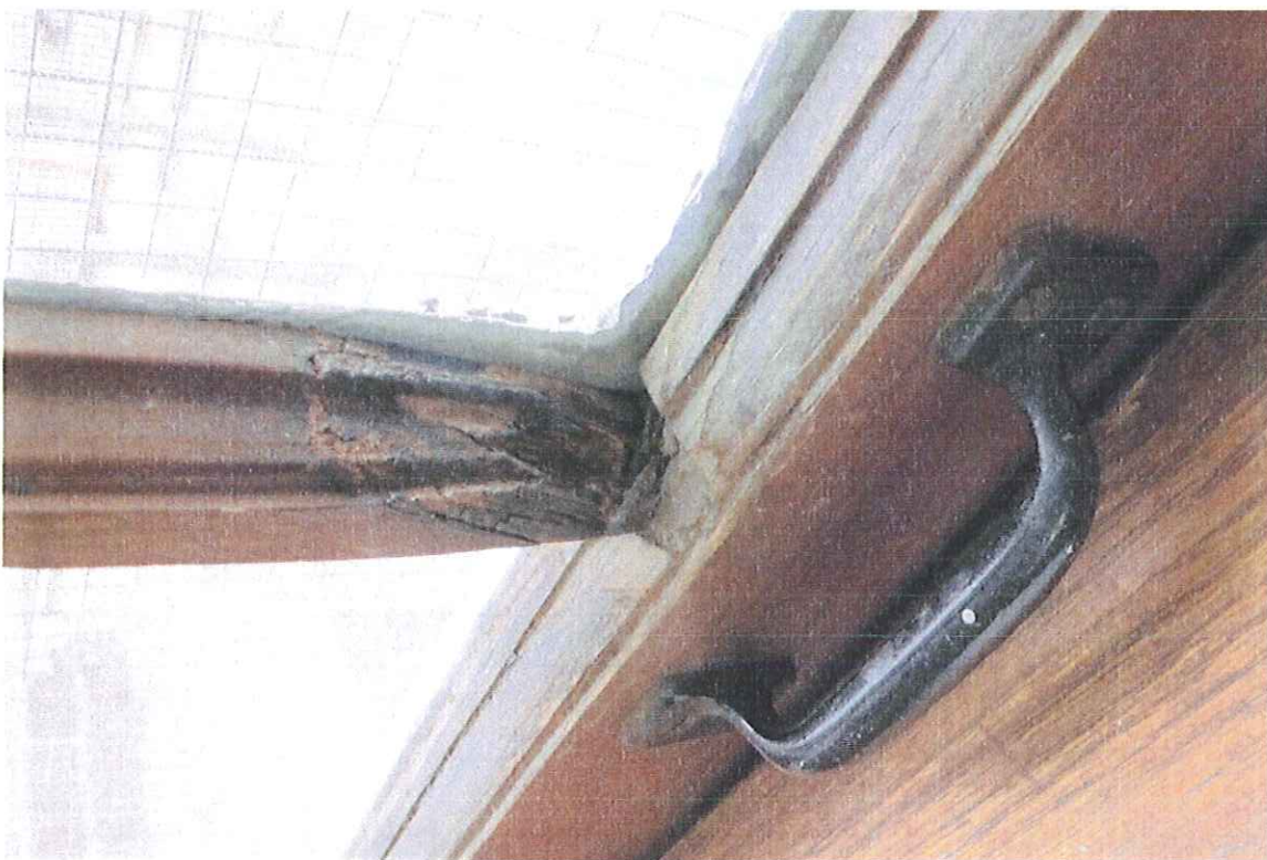
Deteriorated muntin West Classroom
