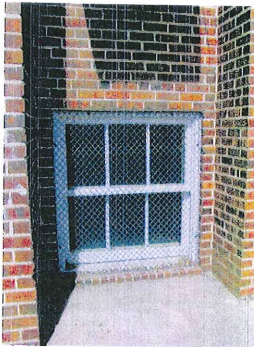
Figure 126: Exterior view of window type C. Note the chain link security screen typical on the exterior of these windows.
