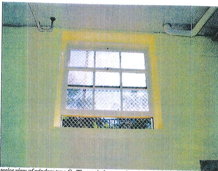
Figure 127: Interior view of window type C. These windows are found along the east elevation of the basement of the original building.
