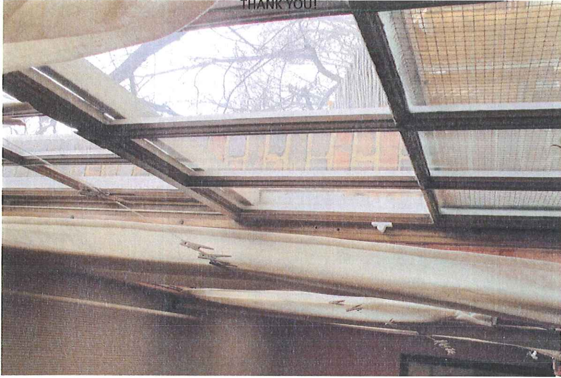
West Facing Classroom - window will not shut completely, exterior peeling paint.
