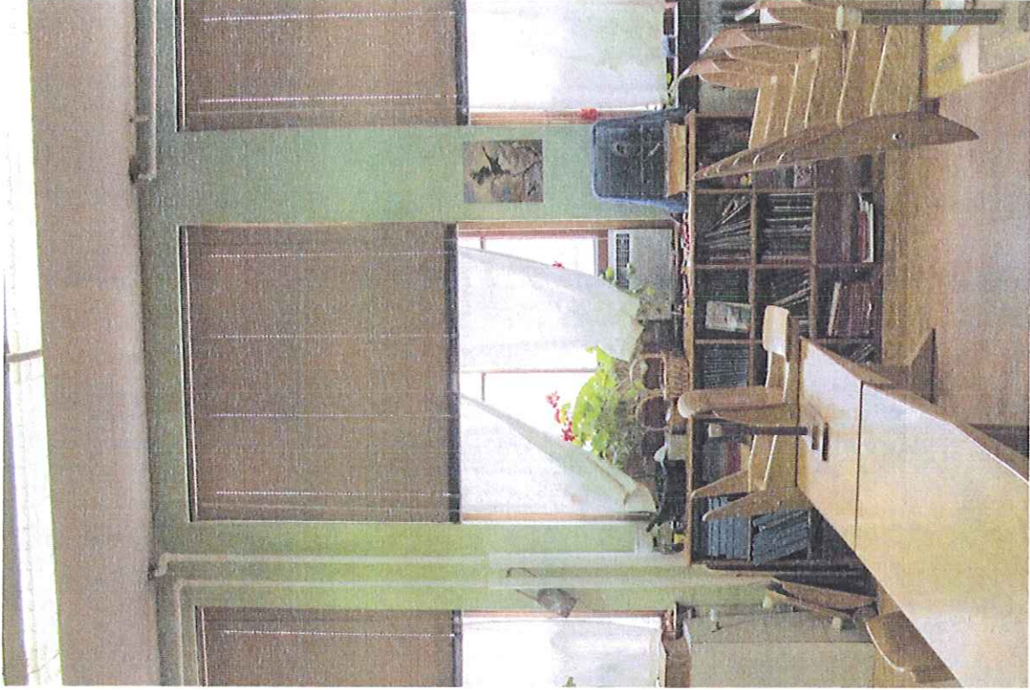
Mini A.C. installed in East Classroom Window
