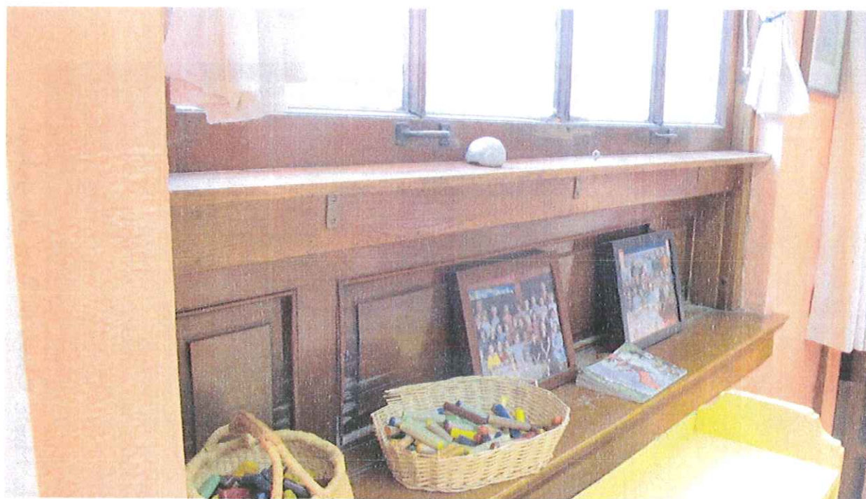
Detail of oak panel, shelf Broken pulley and sash cord
