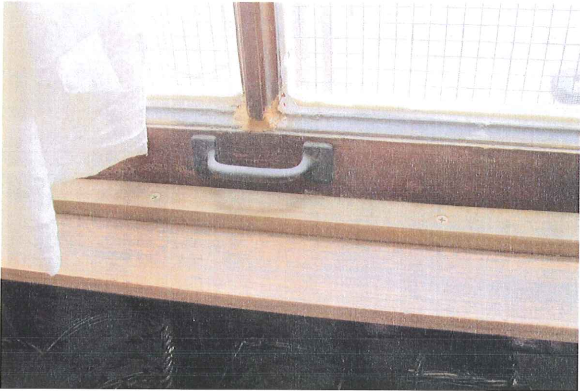
Damaged Muntin, trim installed to "seal gap" between bottom rail & sill West Classroom, Level One
